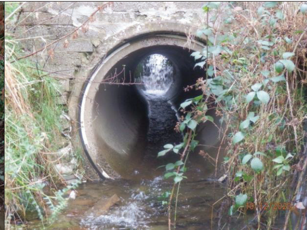
View of culvert outlet ca. 55m u/s of outlet. Note the impassable falls at the upper end of the culvert.
